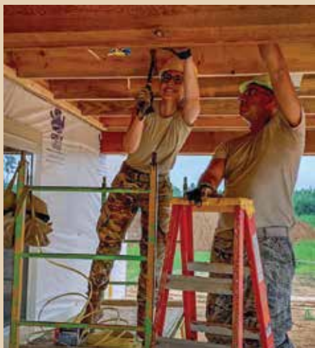
Airmen with the 108th and 177th Civil Engineering Squadrons install electrical circuits on a cabin porch at Camp Kamassa, Aug. 1, 2019. (U.S. Air National Guard photo by Capt. Nathan Gorey)
