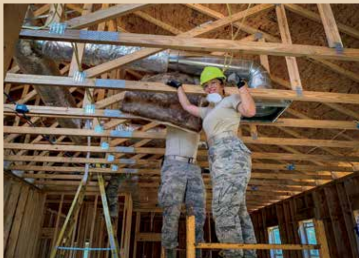
U.S. Air Force Airman Destiny Carl, 177th Civil Engineering Squadron, installs insulation wrap on a heating, ventilation, and air conditioning duct at Camp Kamassa in Crystal Springs, Miss., Aug. 1, 2019. (U.S. Air National Guard photo by Capt. Nathan Gorey)
